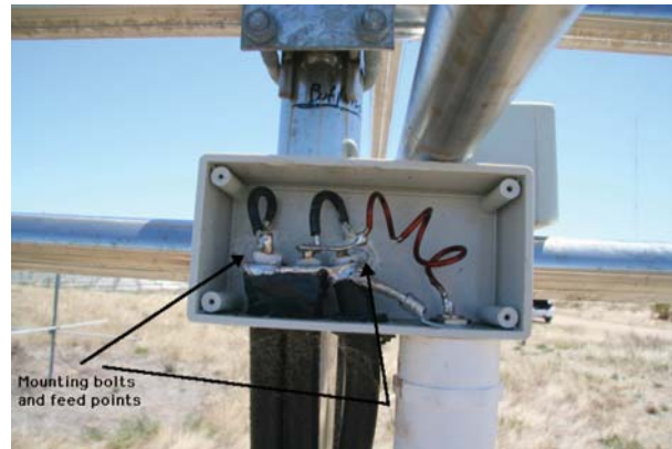
Figure 4.12: Close up of the balun mounted via 2 bolts that connect directly to the feedpoint. Photograph by Daniel McIntosh.
